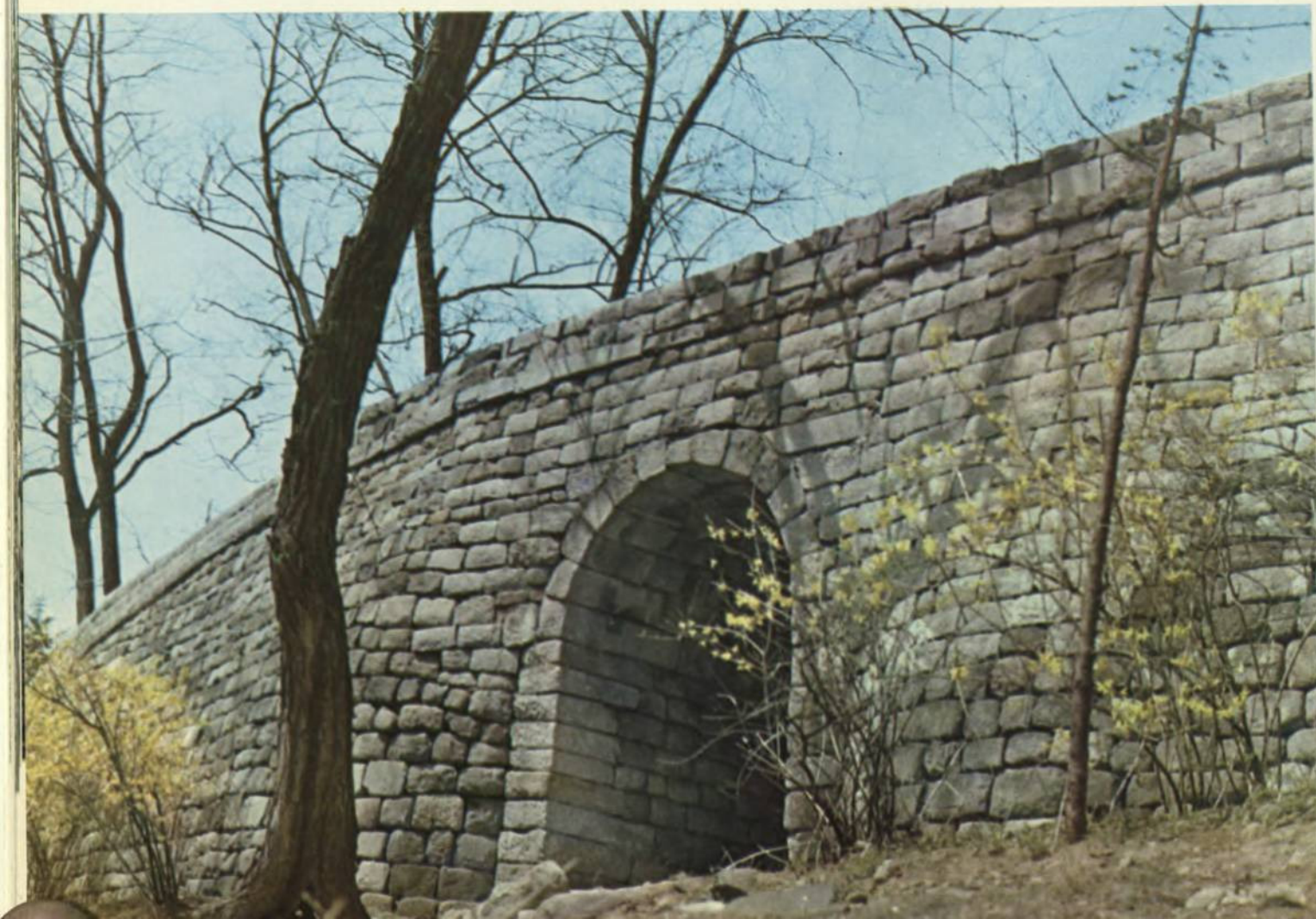
The Tongam-mun Gate, eastern emergency gate of Naesong (inner town), the Pyongyang Walls
