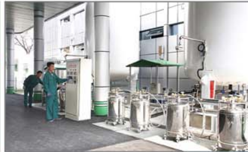
Liquid oxygen filling station.
